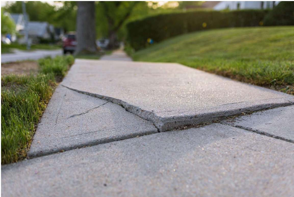
Figure 4: Heaving Concrete (Source: Foundation Supportworks)
